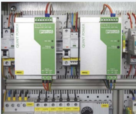
Power supply protection
